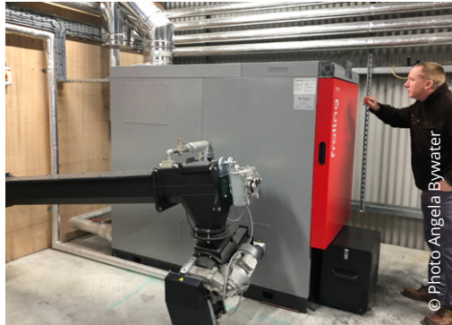
Figure 7: Biomass boiler with feed system
